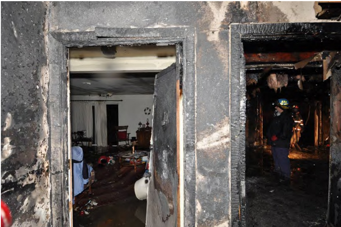
This picture depicts the effects a fire has on rooms with an open door and a closed door.
